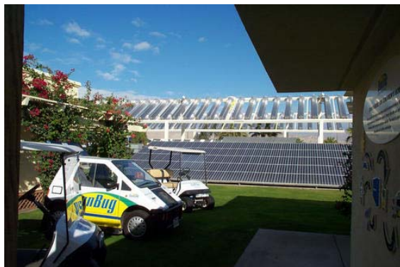
Solar-powered electrolysis system at SunLine Transit Agency
